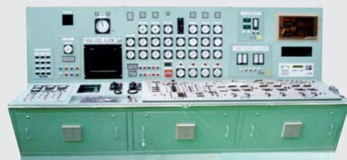
Control console & Mimic panel
