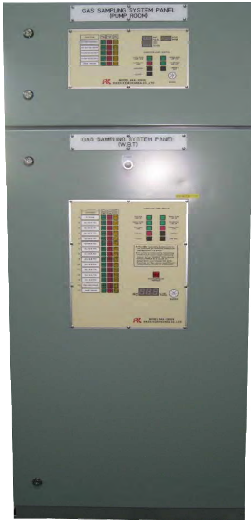
For Pump Room
